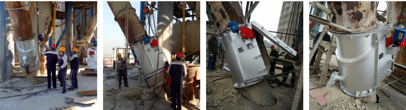
Shandong Tai'An Zhonglian Cement Co.,LTD Field installation scene of Preheater Flap Valve
